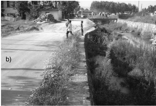
Figure 4. (a) Survey of a flood control canal constructed with concrete and stone at site 6. (b) Photograph of west wall of canal. Note the linear nature of the inside edge of the wall that we surveyed and the warping and displacement at the main fault.
