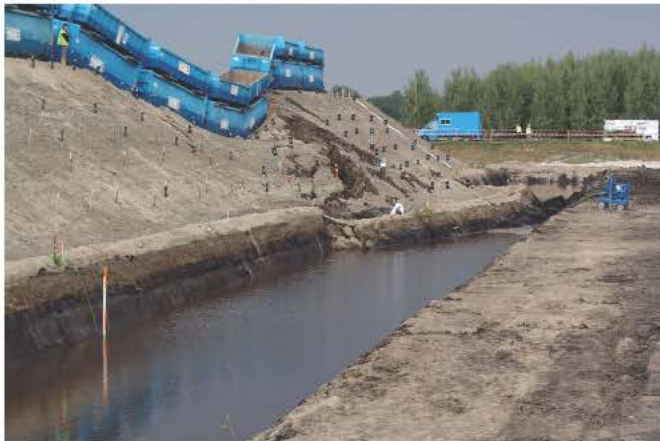
Fig. 3. Example of a physical model of a river dike taking a 1:1 approach ( http://www.dijkmonitoring.nl/en/projects/ ).
