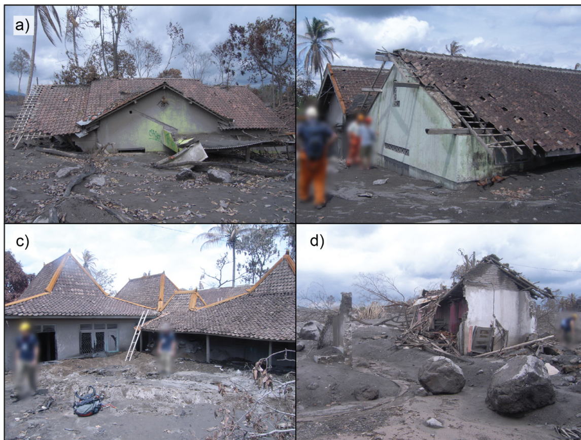
Fig. 3. Photos of slow overflow flow impacts in Bakalan village including: a) Thick deposits of up to 2.5 m partially burying houses and causing structural damage on upflow side of structure, b) inundation with minor structural damage, c) flows blocked by building fronts, resulting in little to no inundation, d) severe structural damage caused by large boulders carried by the dense flow. Photos taken 7 December 2010 by S.F. Jenkins.
