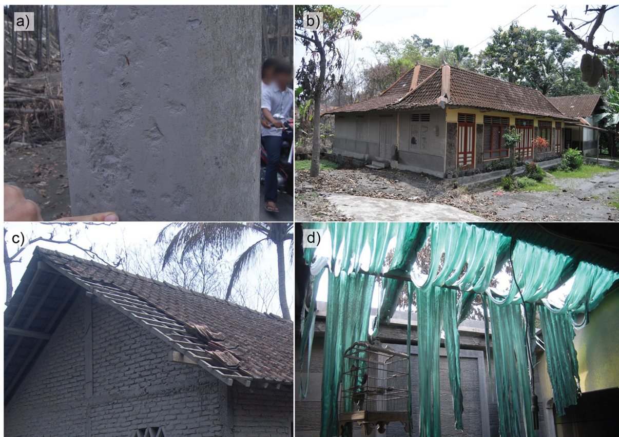
Fig. 7. a) ~7.5 m high concrete utility pole at the base of the concrete levee bordering the Gendol channel showing pockmarks on the upflow side, from small clasts carried within the Leds striking the pole; b) Traditional Javanese building at the edge of Bronggang village showing the very sharp Leds boundary, with ash and dried vegetation from the Leds visible on just the upflow (left of image) wall and surrounds; c) Roof tiles lifted on the overhang of a building facing the direction of Leds overspill suggesting dynamic pressures of ~0.1 to 0.2 kPa; d) Corrugated plastic roofing sheets melted by the Leds and/or the deposits suggesting temperatures of at least 100 °C sustained for ~three minutes. Photos taken by S.F. Jenkins, November 2010.
