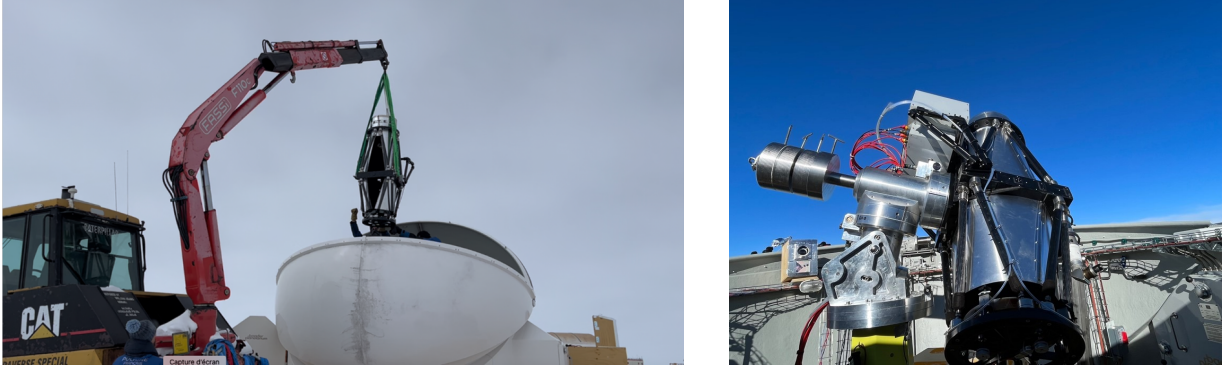
Figure 6. Left: Installation of the ASTEP+ telescope in its new dome, using the logistical means of the station. Right: The ASTEP+ telescope equipped with its new focal box fully installed in the new dome.
