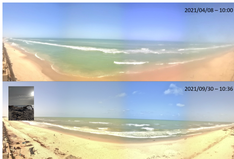
Figure 2. Images acquired with the camera (see Figure 1 for location) on the indicated time. A small picture (bottom panel, on the left) shows the on-going construction of the riprap.
