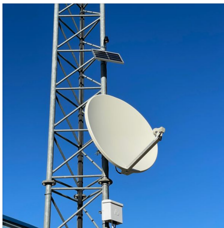
Figure 2. Image of a sensor installed by HD Rain on a mast of a fire brigade building (commercial collaboration with the SDIS, departmental fire and rescue service) with in the south of France
