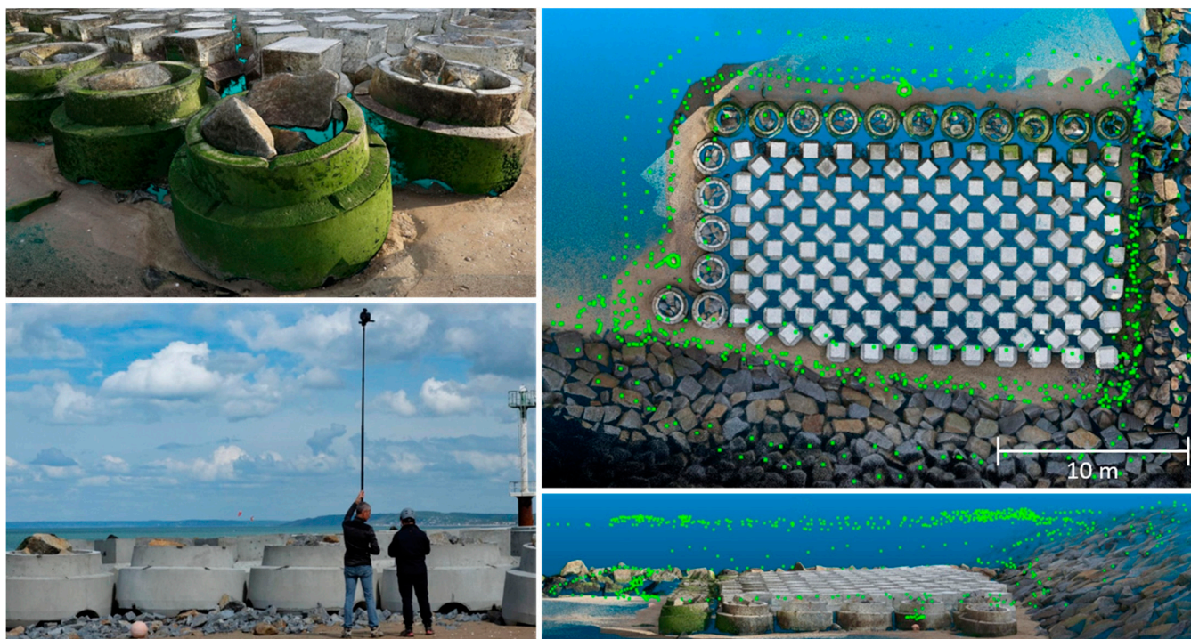
Figure 5. Studied object: Armor blocks (top-left), photogrammetric survey (bottom left), overall site and photo positions (top and bottom right).
